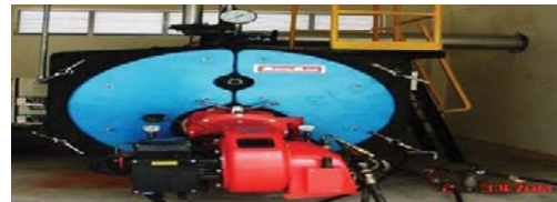
Figure 2. Boiler for steam generation [6]
