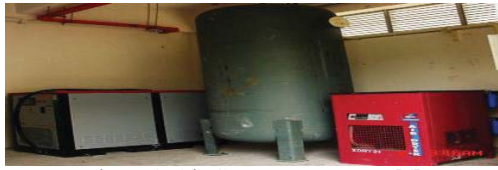
Figure 3. Air Compressor Room [6]
