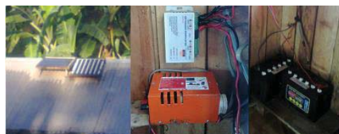
Figure 4. Typical Solar Home System (Panels, Charger controller, Inverter and batteries)
